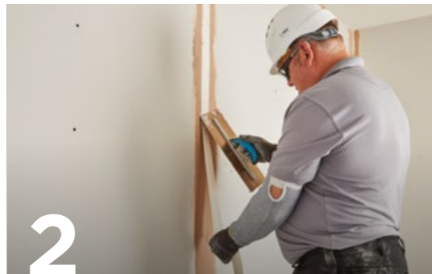
2 Where there is an increased risk of cracking, or where gaps exceed 3mm, the gaps are reinforced with Gyproc Joint Tape bedded in Thistle plaster. In other situations, plasterboard joints can be reinforced with Thistle ProTape FT50 or FT100 glass fibre mesh tape.
