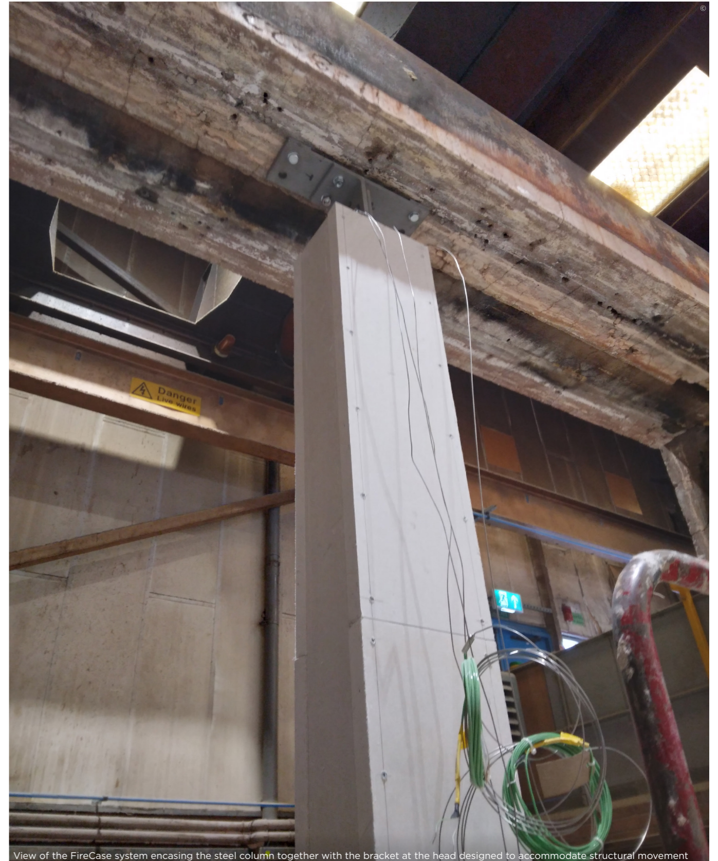
View of the FireCase system encasing the steel column together with the bracket at the head designed to accommodate structural movement
