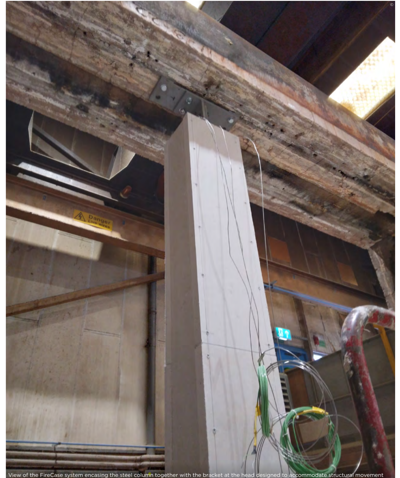
View of the FireCase system encasing the steel column together with the bracket at the head designed to accommodate structural movement
