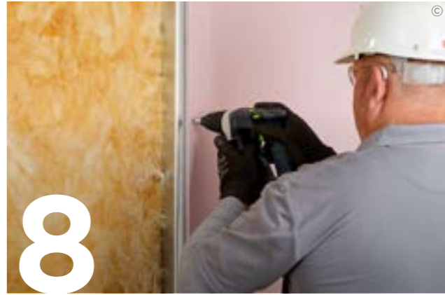
8 Use British Gypsum Jackpoint Drywall Screws to fix Gyproc plasterboards or Glasroc specialist boards to the SFS framework.
