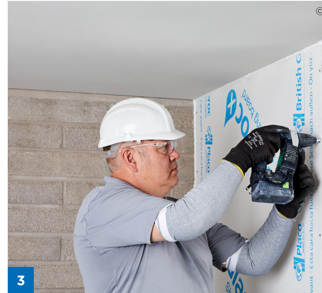
Use Glasroc X Screws 25 mm to fix Glasroc X Sheathing Board to the SFS framework.
